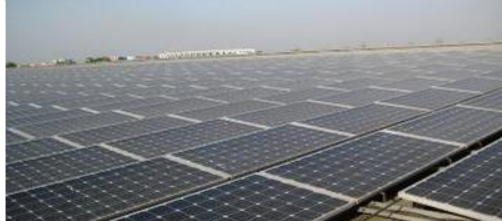
Rooftop 1 MW Grid Integrated Solar PV*
