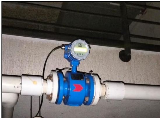
Water meters for Domestic water (treated lake water), HVAC & treated water for irrigation
