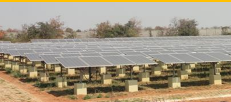
Solar Farm in IMGEOS & NDEM Facility of ISRO, Shad nagar, IGBC Platinum
