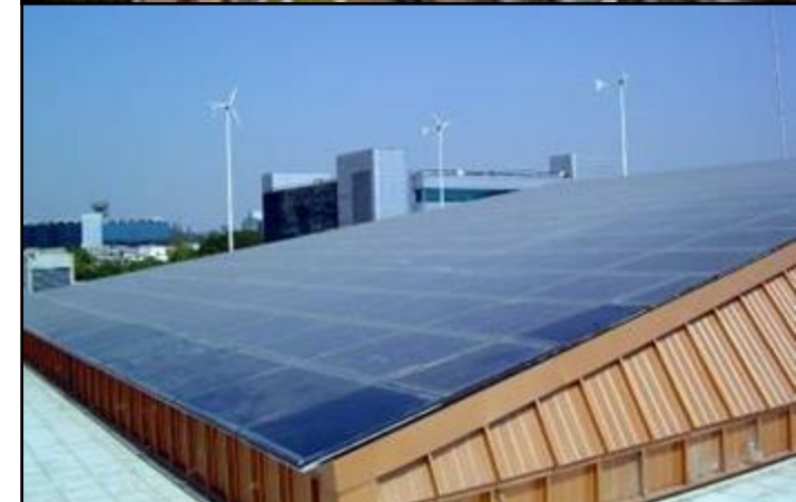
Micro Wind Turbines -Suzlon One Earth, Pune -IGBC Platinum
