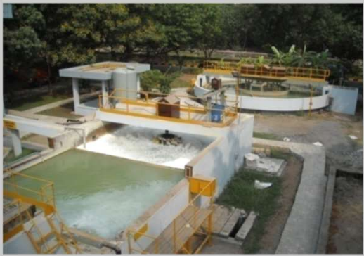
Zero Liquid Discharge Facility (1 ETP & 5 STP)
